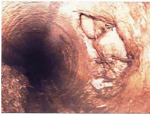
(c) 管道腐蚀
